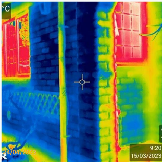
Thermogram showing heat loss through brickwork
