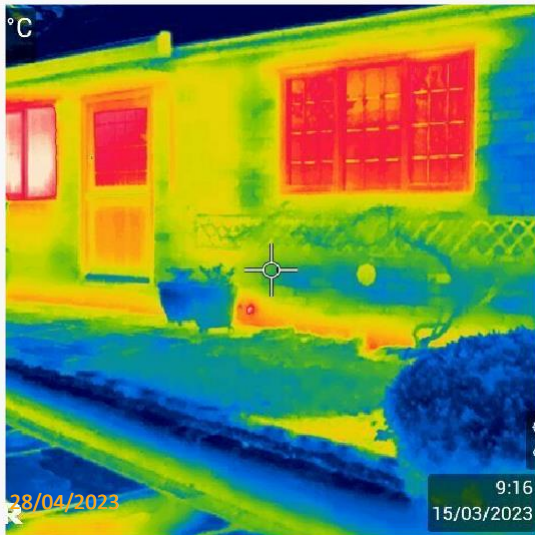
Heat loss from floor slab and door
