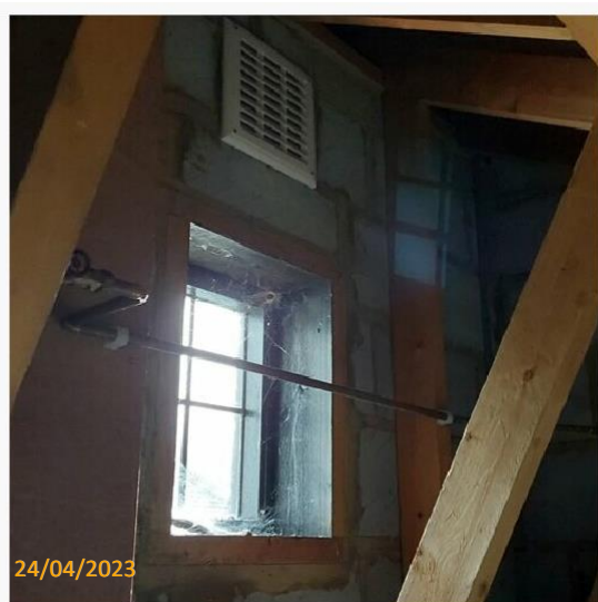
Ventilation required in the roof void
