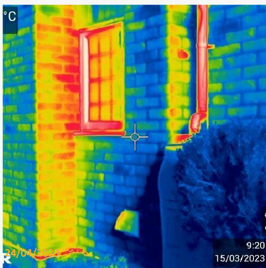
Thermogram showing heat loss through brickwork
