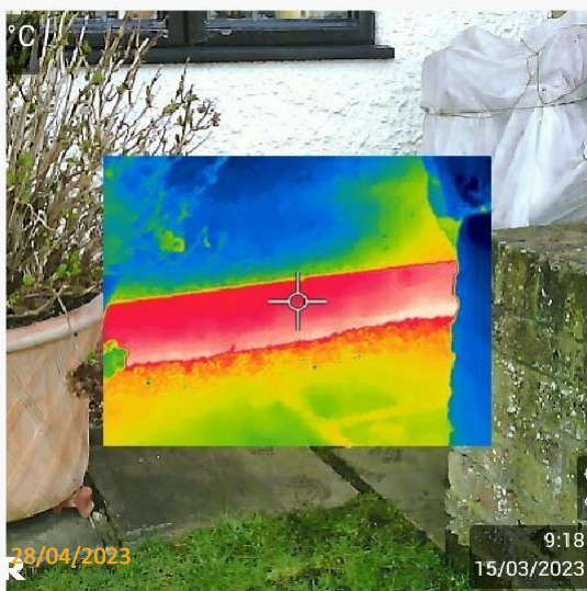
Heat loss from floor slab
