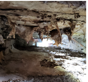
Avoid water damage
