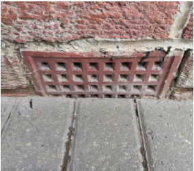
No blocked air bricks
